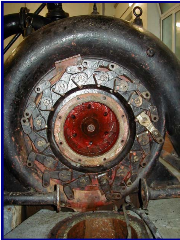
* Interior Turbina Francis
